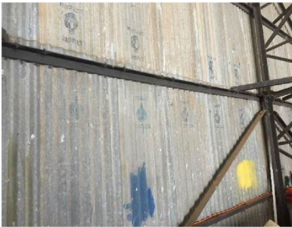
Figure 3.21 Lysaght Orb blue stamped galvanised corrugated steel on interior steel framing. (Source: GML, 2018)
