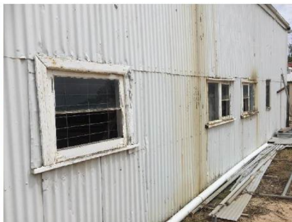
Figure 3.16 Eastern side of Hangar No. 1 showing timber windows in poor condition. (Source: GML, 2018)
