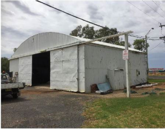
Figure 3.11 Front (ie openable side) of Hangar No. 1 showing outrigger doors. (Source: GML 2018)
