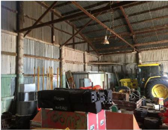
Figure 3.13 Interior of Hangar No. 1 showing framing structure including raw timber log posts. (Source: GML, 2018)
